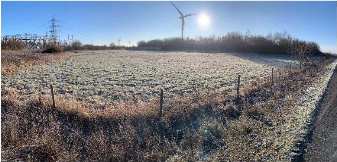
Position 19: Small grassland area at the substation
